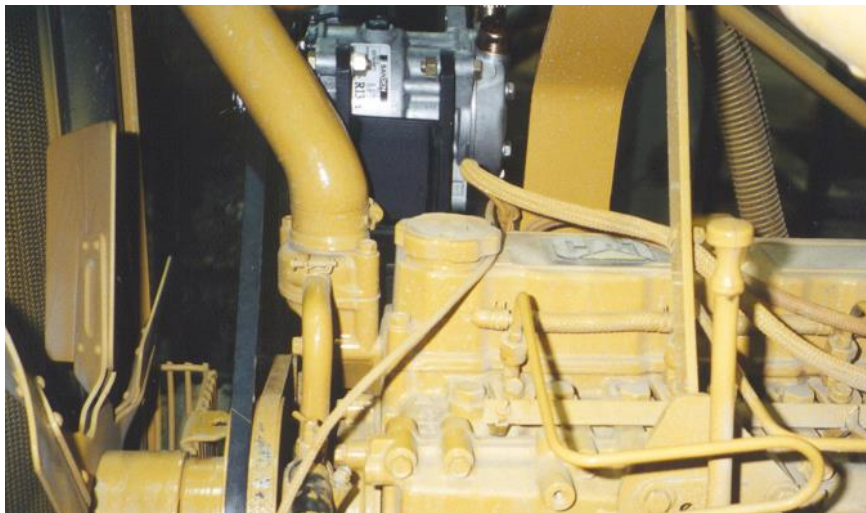
Back view of compressor assembly.
